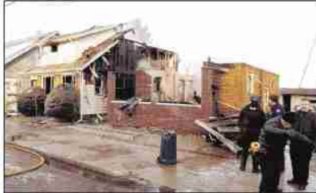
The home at the 1100 block of West 25th Street was destroyed by the early Tuesday morning fire.
